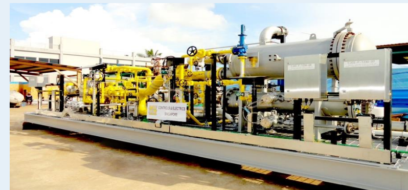
Chemical Injection Skids
