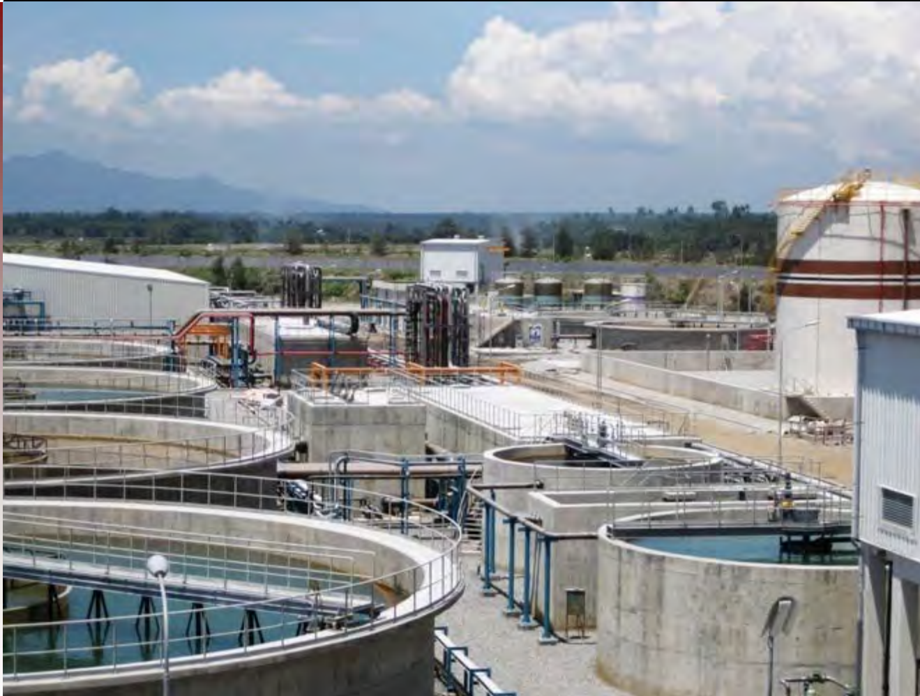
Tanjung Jati B Seawater Desalination Plant INDONESIA
