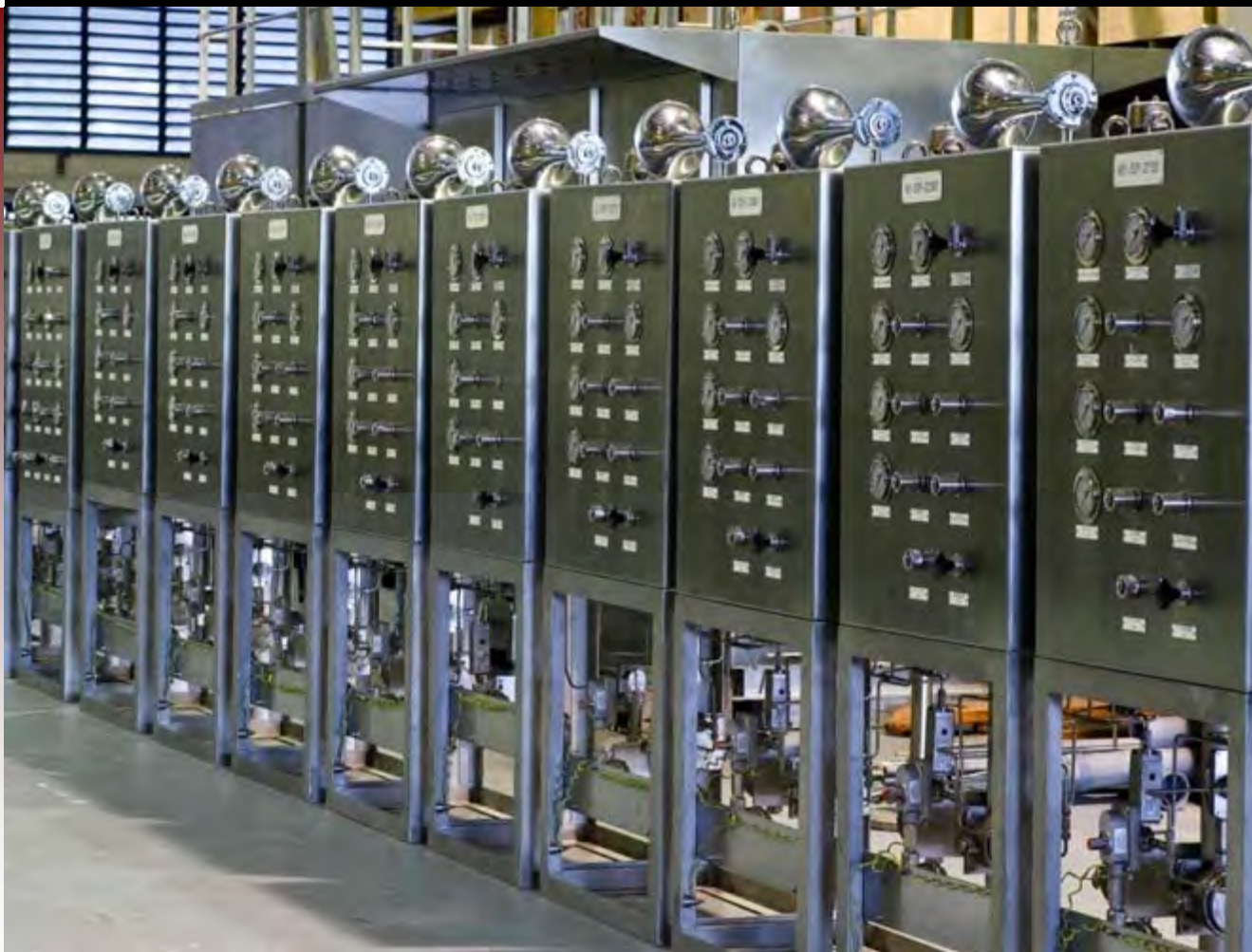
Wellhead control panels INDIA
