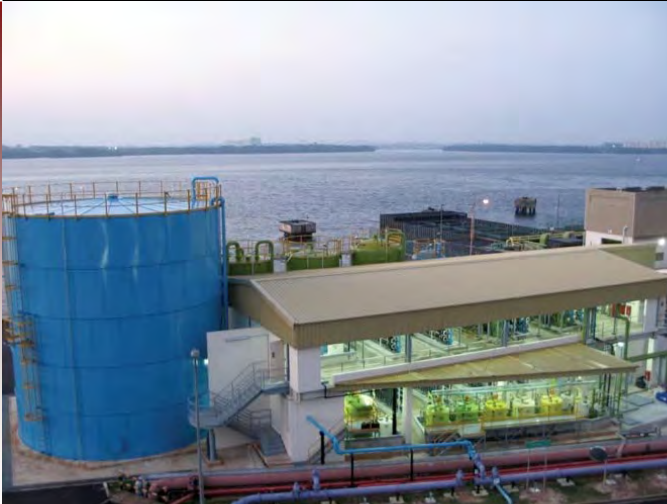
Senoko Power Station Seawater Desalination Plant SINGAPORE
