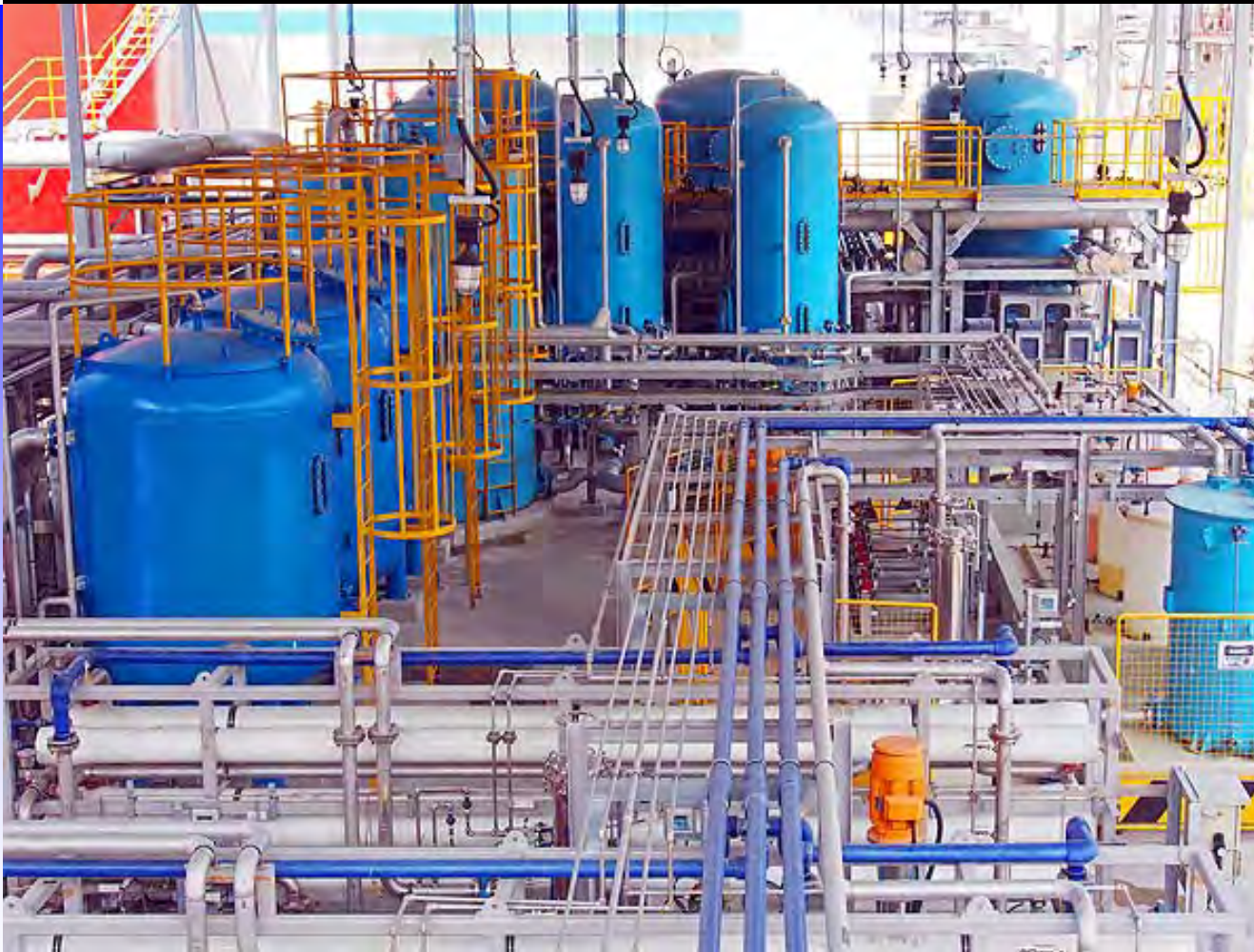
Tembusu Multi-Utilities Complex Plants SINGAPORE
