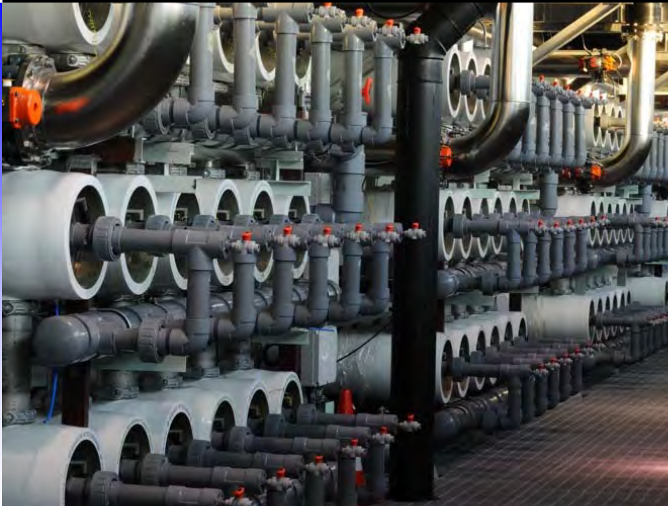
Bedok NEWater Factory Phase II SINGAPORE
