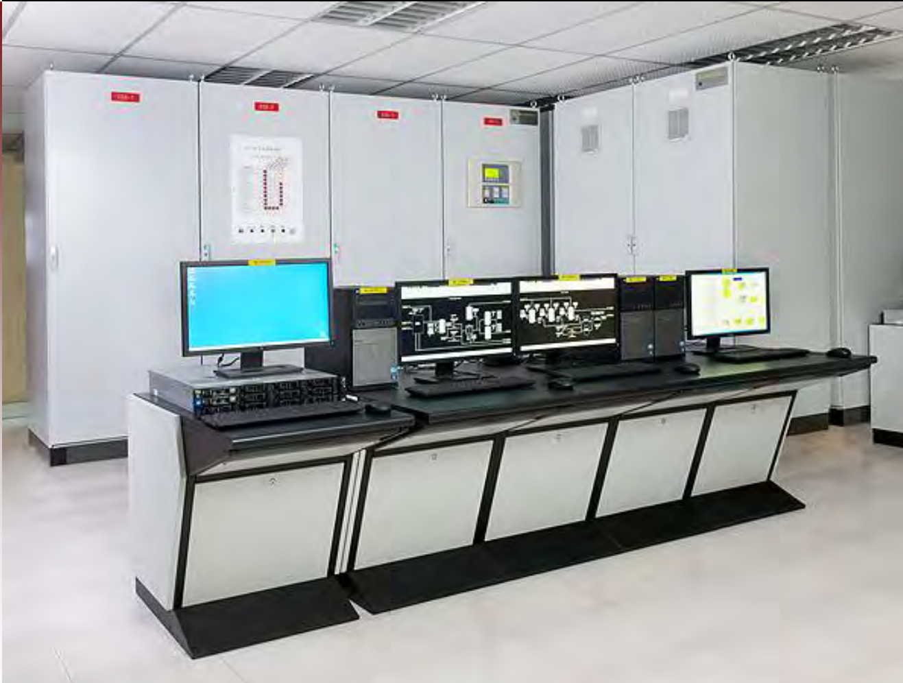
Emergency shutdown system VIETNAM
