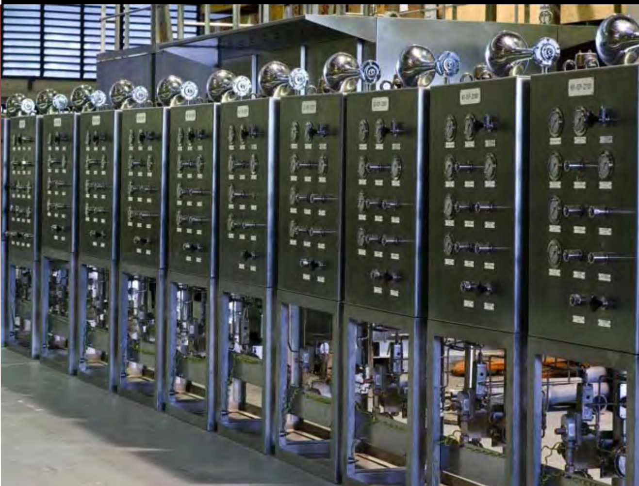
Wellhead control panels INDIA
