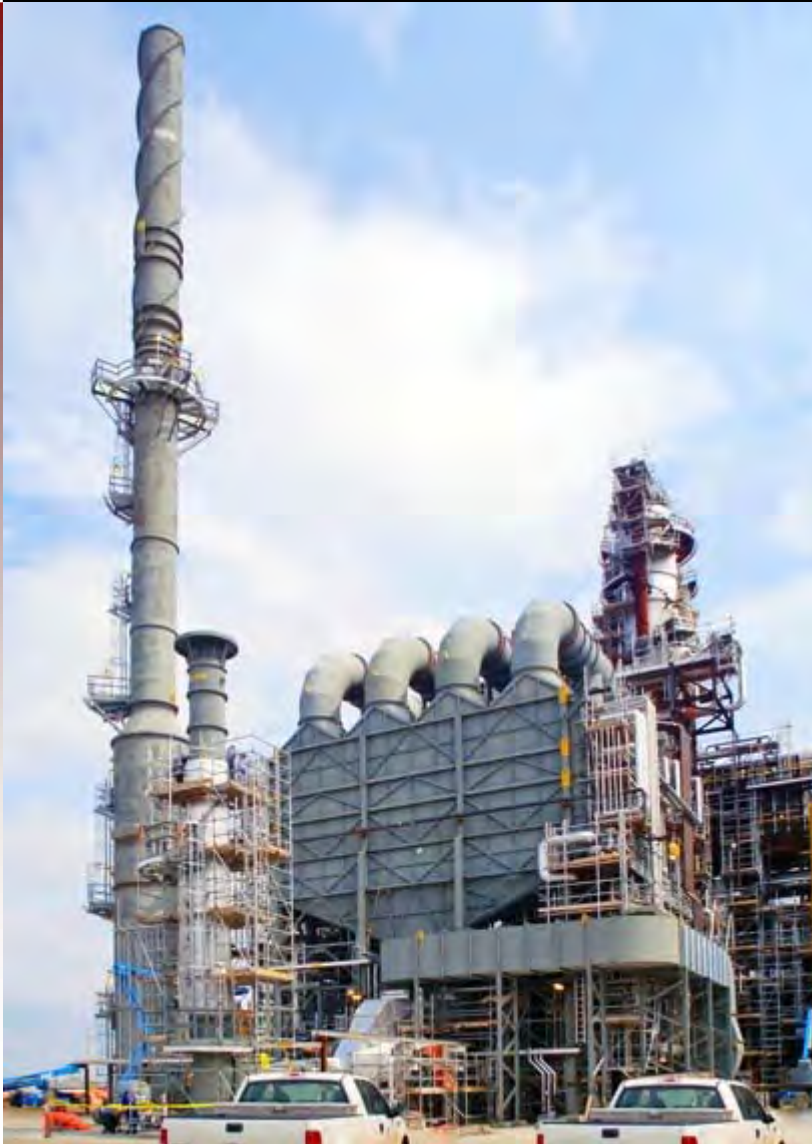
Oil sands upgrader CANADA
