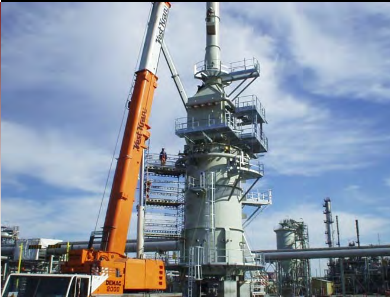
Reactor effluent furnace NORWAY
