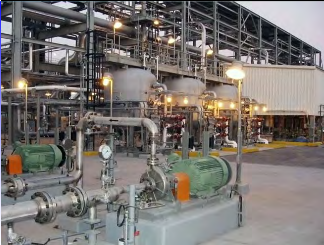
Hawiyah NGL Reverse Osmosis Plant SAUDI ARABIA RO plant at Saudi Aramco's largest NGL processing plant
